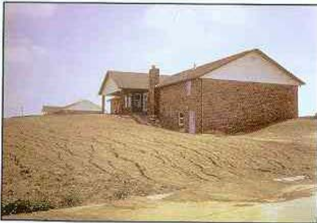
Uncontrolled erosion degrades water quality and costs time and money to repair.
